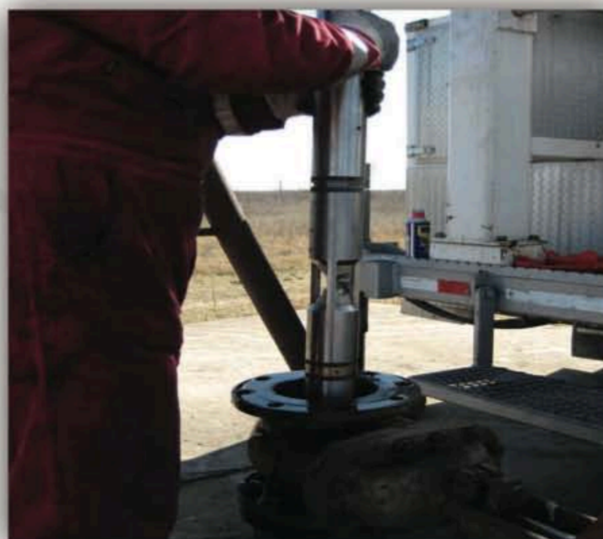
AST Firing head being lowered into well for cross well operation, Devine Well, Texas 2011
